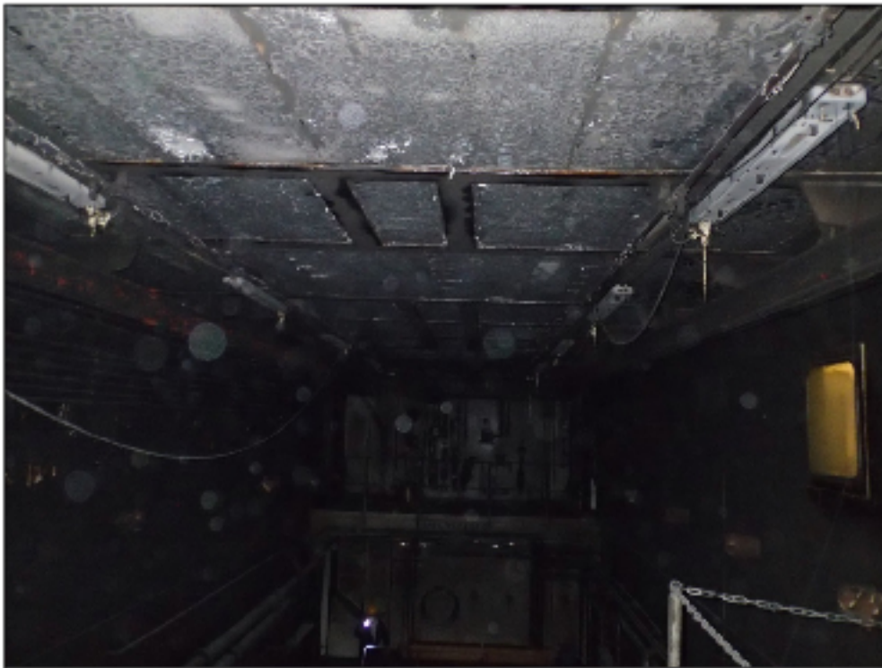
Figure 7: Traces of fire in the engine room
