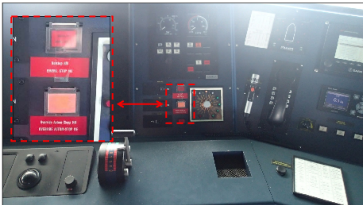
Figure 24: Override pushbutton in the control console on the bridge
