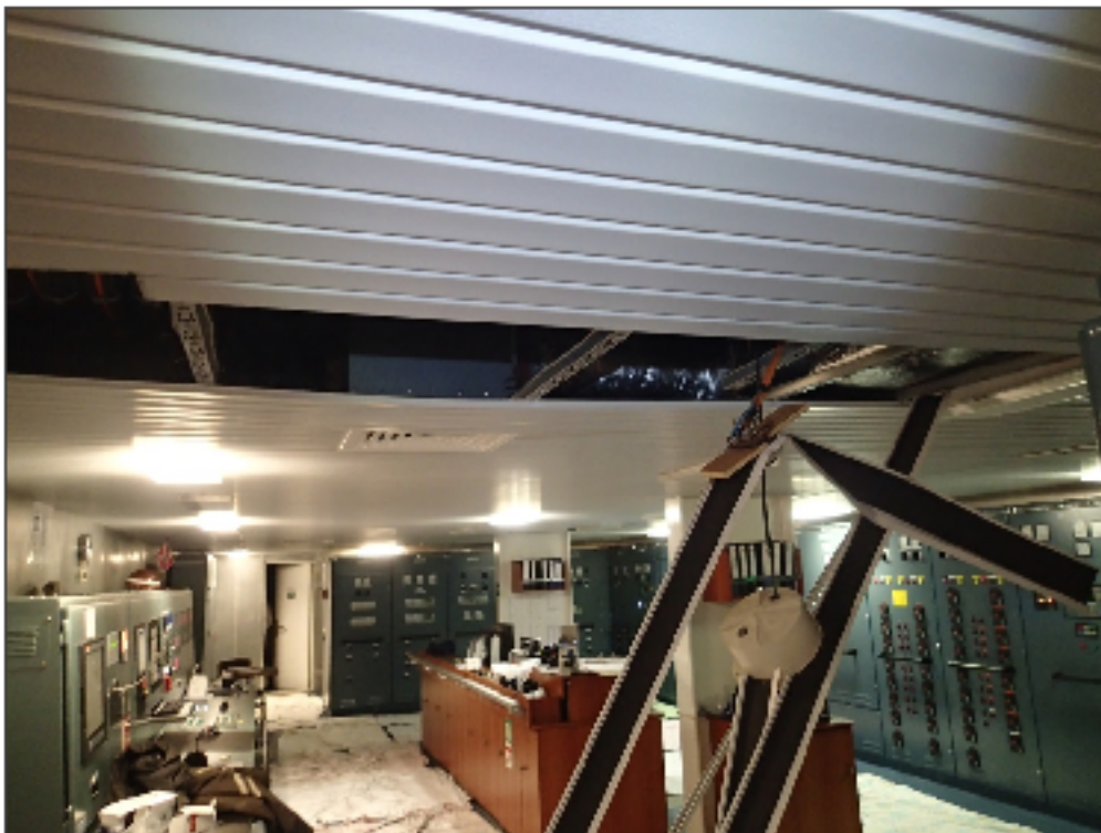
Figure 8: ECR with detached ceiling lining
