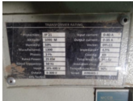
Figure D.36.21 Transformer (Traced: Manufactured in IR)
