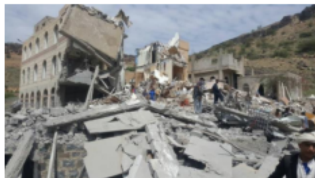
Figure B.58.4 Post-blast damage
