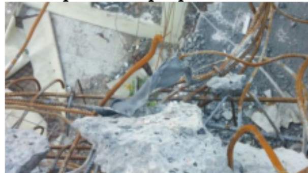
Figure D.60.5 Civilian apartment complex post blast
