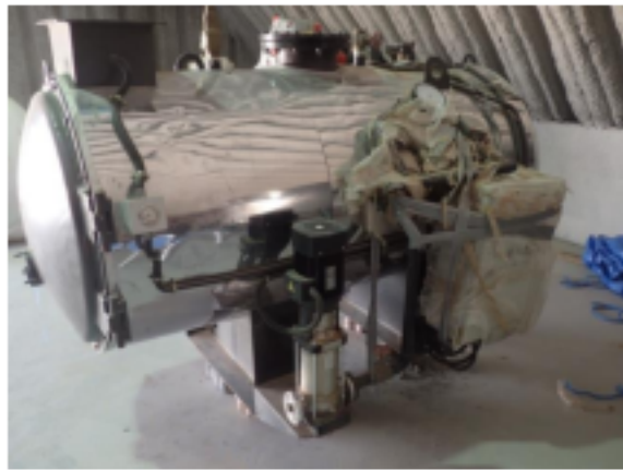
Figure D.36.6 Pressure vessel
