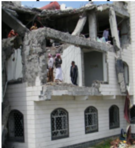
Figure D.60.4 Civilian apartment complex post blast
