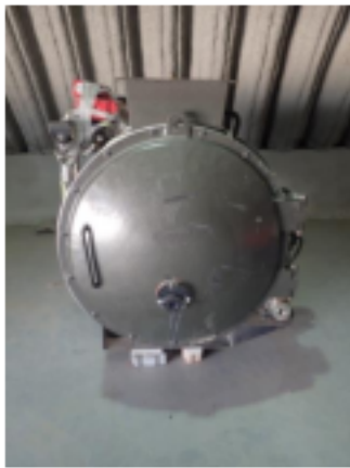
Figure D.36.5 Pressure vessel
